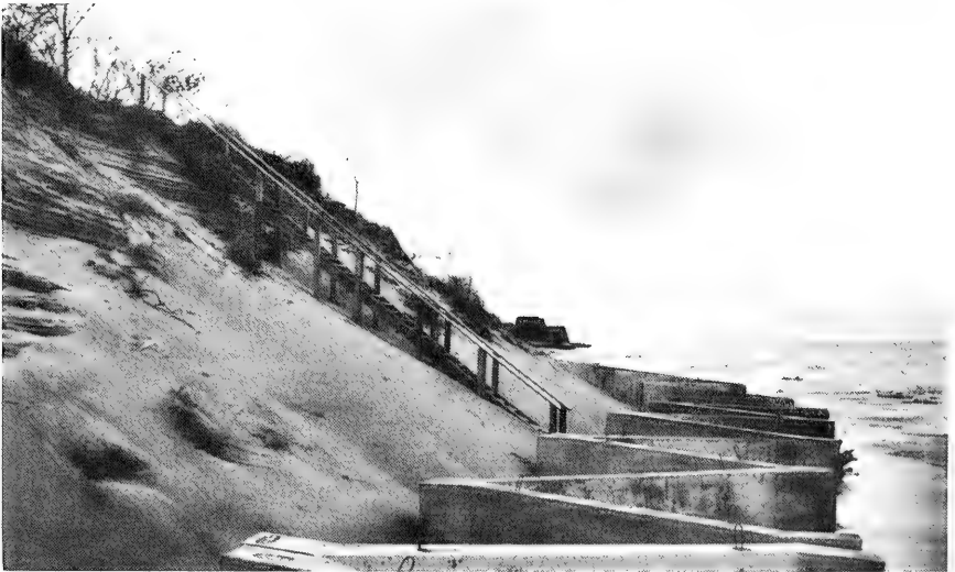
Figure 18. Bluff at CERC profile line 16 recently stabilized by precast-concrete seawall following a period of severe erosion (16 October 1976).
